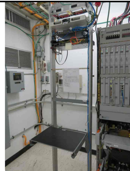
C EXISTING AUX EQUIPMENT RACK
