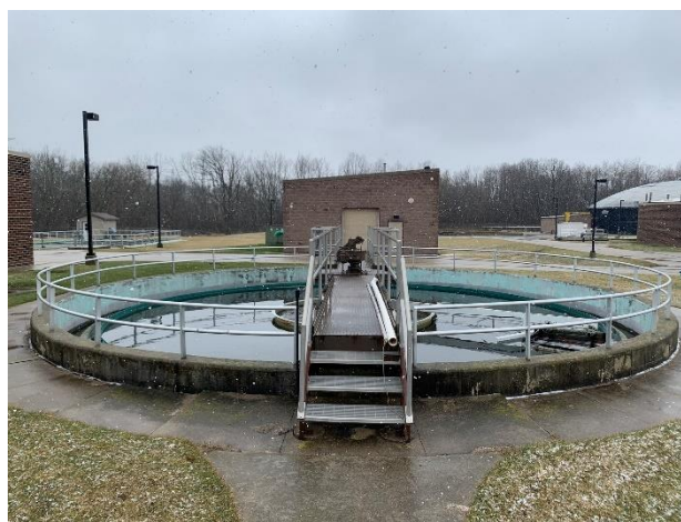
Final Clarifiers – Original
