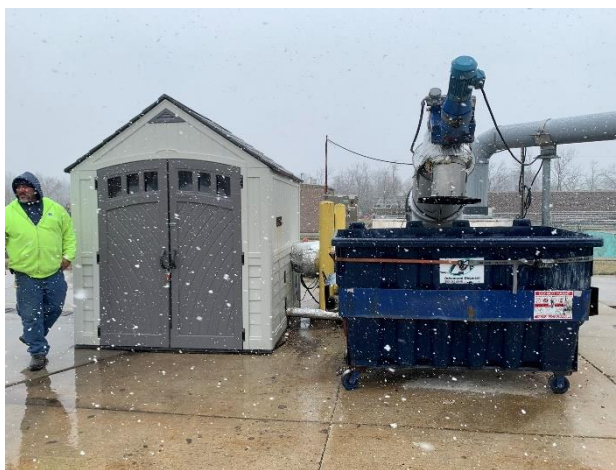
Waste Receiving Station
