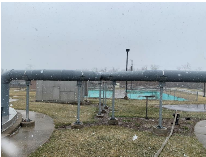
Odor Control Unit
