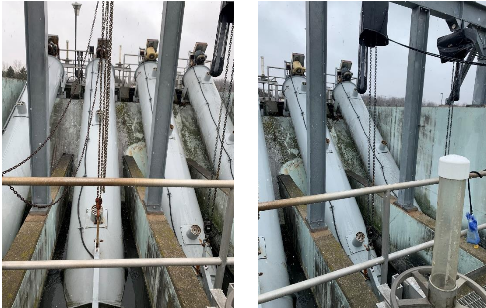
RAS Pumping Station w/ Archimedes Screws
