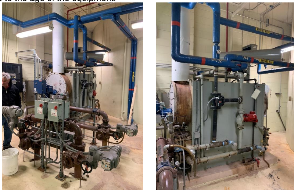
Boiler / Heat Exchanger
