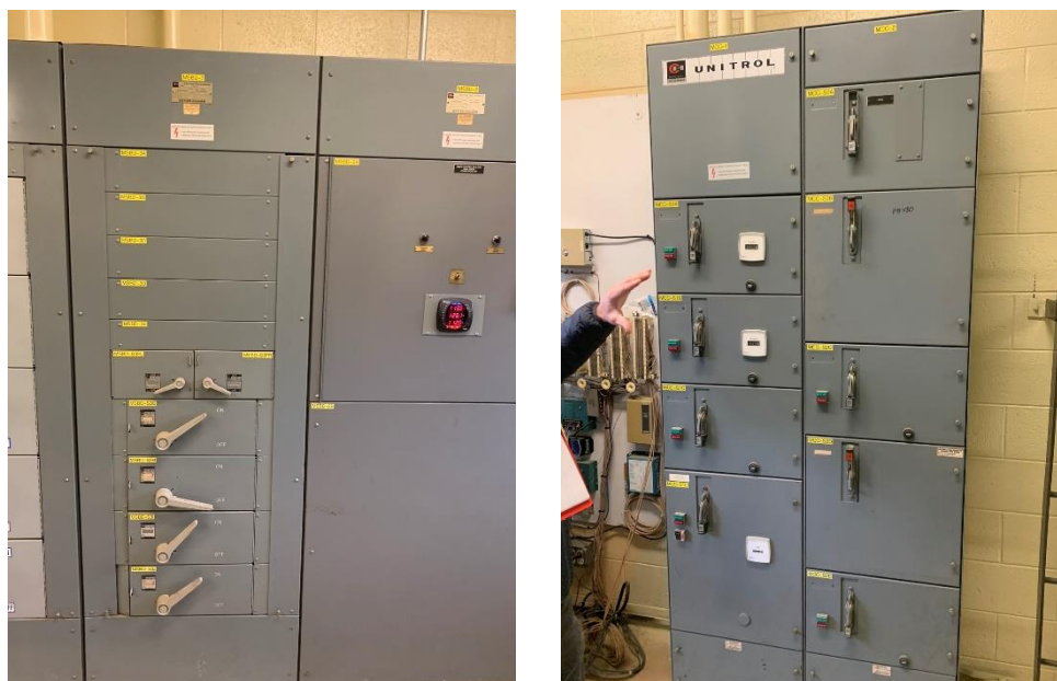
Electrical Room - MCCs
