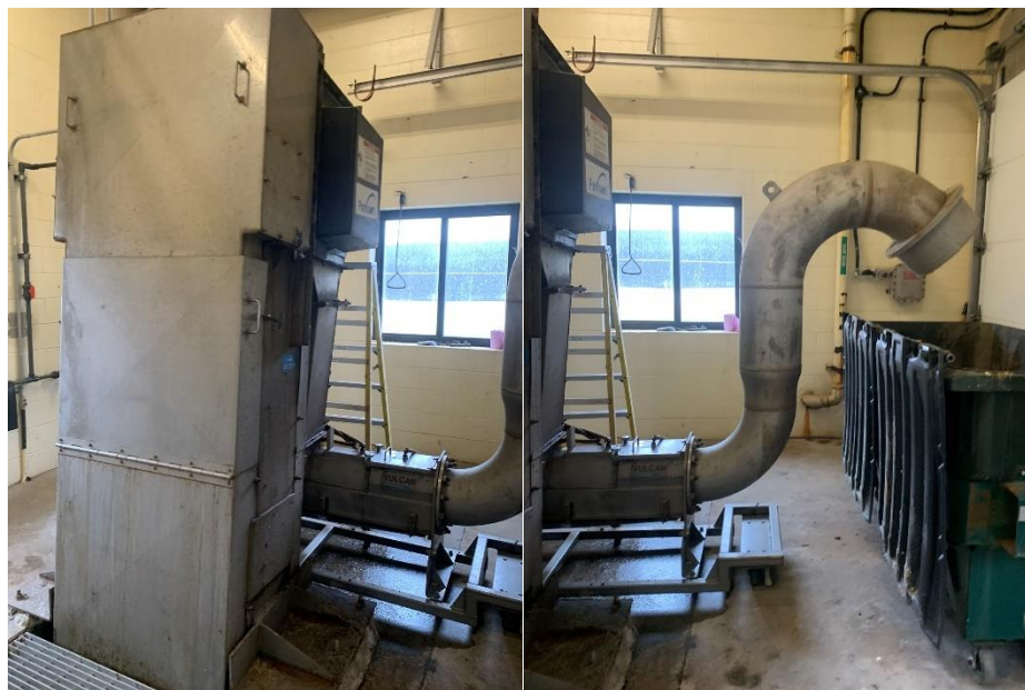
Screen and Screenings Washer / Compactor
