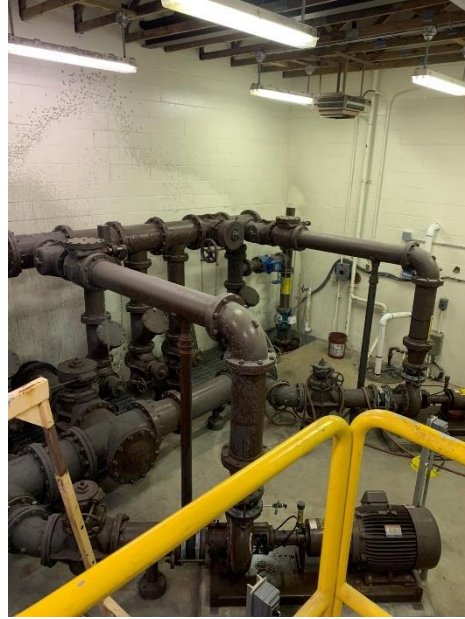
Pumps and Piping
