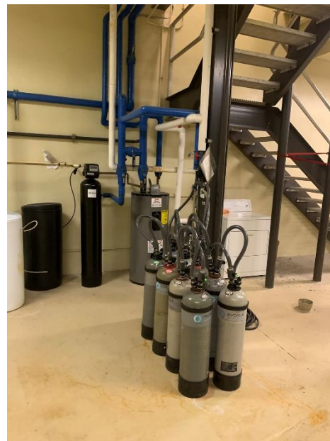
Reverse Osmosis Equipment
