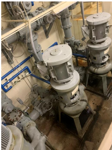
RAW Pumping Area
